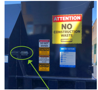
Compactor Hutch With Safety Interlock
