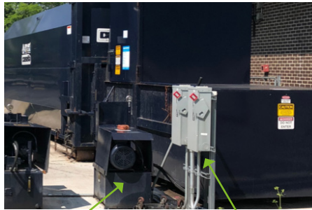
Compactor Power Unit with Emergency Stop Button
